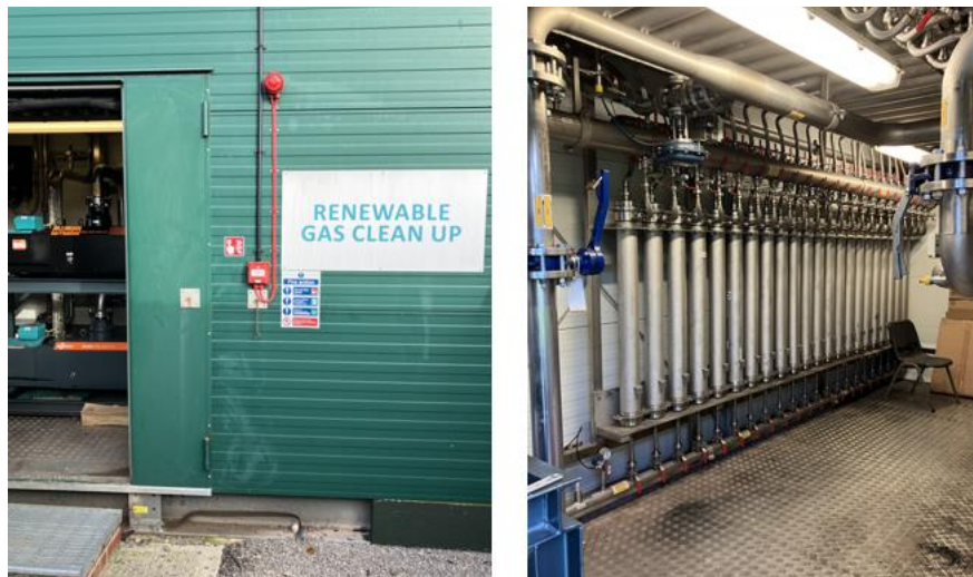
Figure 8 – Gas cleansing membranes converting raw biogas to biomethane
